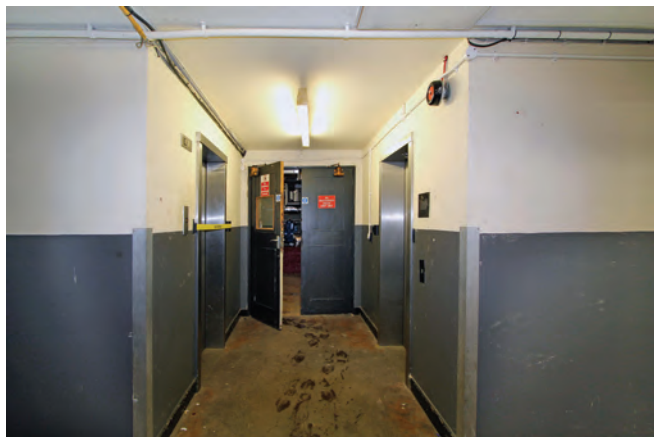
The town hall lifts (seen left and right) go down to the basement. The emergency centre is behind the photographer. The plant rooms for the Town Hall are through the wooden doors
